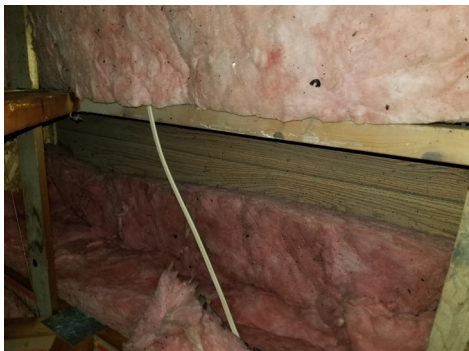
Attic insulation before: low levels of old fiberglass batt insulation in this house were not doing a good job keeping our client warm.
