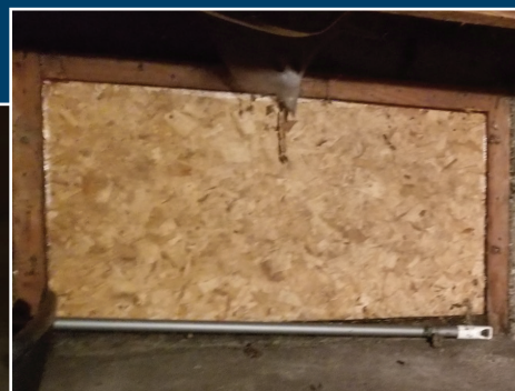
Right: Foundation wall before: bare basement walls allow cold to seep into this Michigan-style basement.
