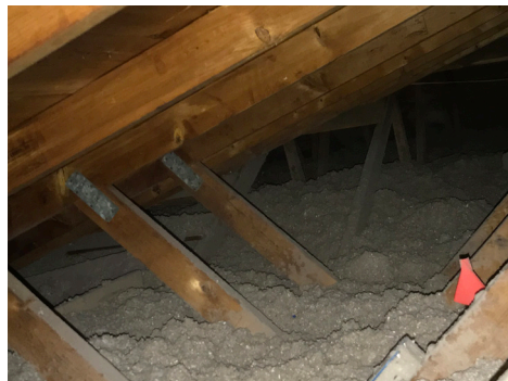
Attic insulation after: blown cellulose insulation, along with air sealing, is more efficient and helps maintain heat in the home with its high R-value.
