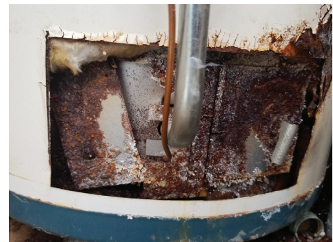
Water heater before: a water heater only lasts about 10-15 years, and this one is well past its life expectancy.
