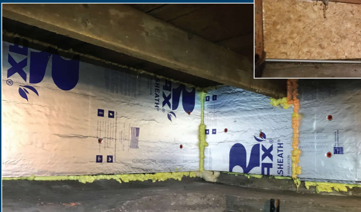
Foundation insulation after: foil-faced insulated boards, air-sealed around the edges, prevent cold from entering the basement in this home.
