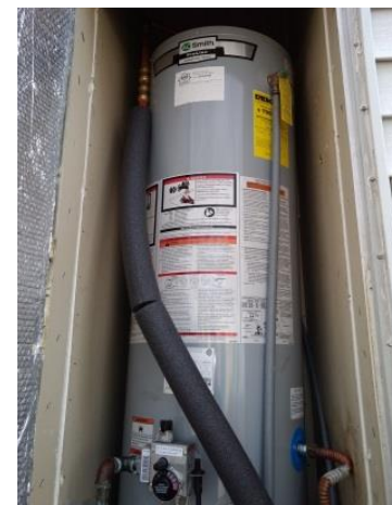
Water heater after: a new, energy efficient water heater will make a big difference in energy costs per year.
