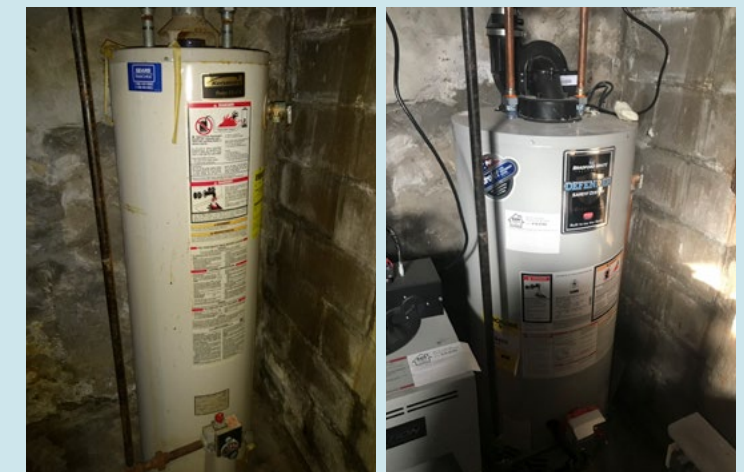
Water heater before and after. A new, energy efficient water heater will make a big difference in energy costs per year.
